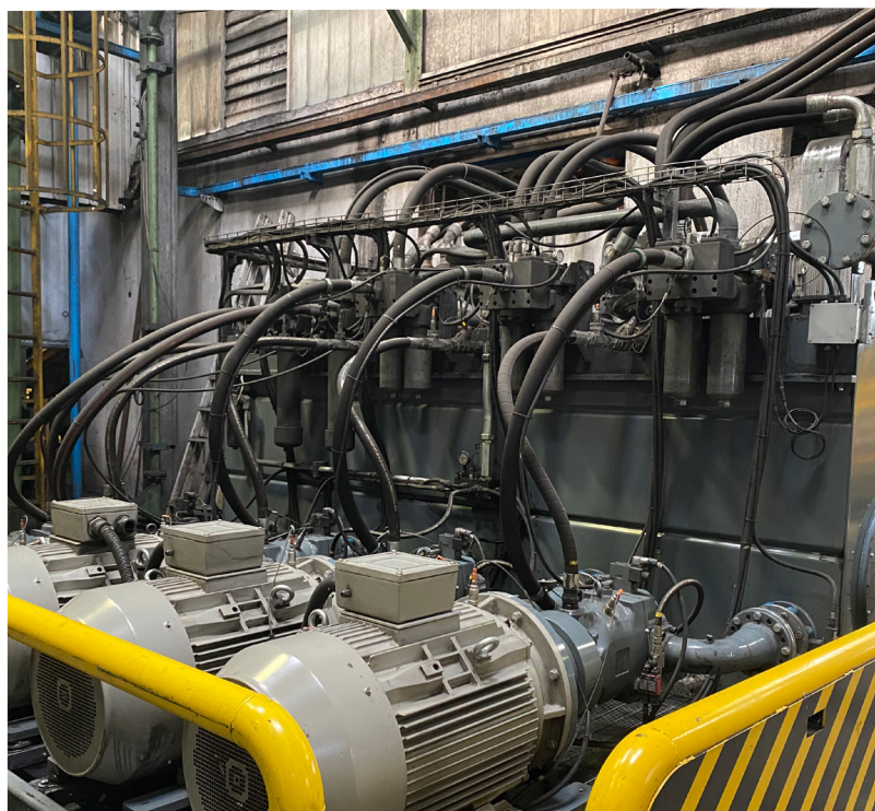
Central moulding plant with integrated diagnostic system developed by Oleobi for Fonderia Ghirlandina
